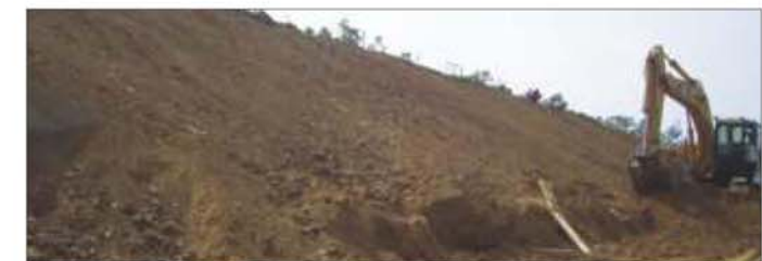
Step 2: Prepare the Site by smoothing & dressing the slopes & removing loose soils & boulders
