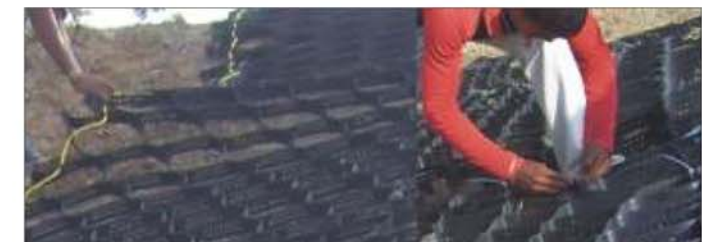
Step 4: Connect the adjoining StrataWeb panels with cable ties. Anchor the StrataWeb geocells with polymer rope tendons and also with 'J'-shaped steel reinforcement bars.
