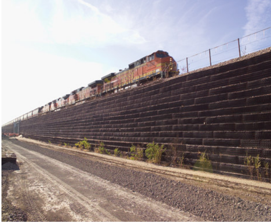
A temporary retaining wall constructed with wire form baskets and geogrid soil reinforcement withstands heavy dynamic loading from 80,000-pounds-per-axle engines.
